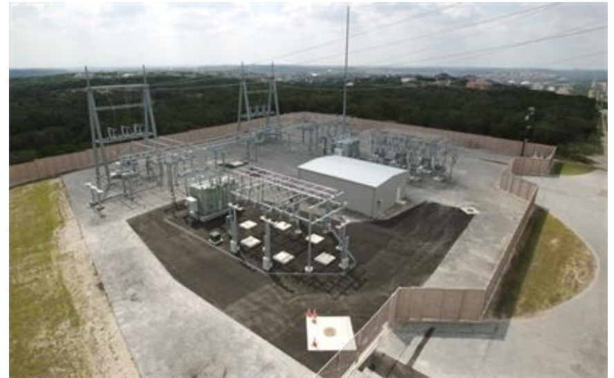
Typical expansion project supported under this type of contract – added a transformer & switchgear in the newly paved area
