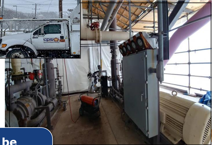
Power Plant Freeze Protection
