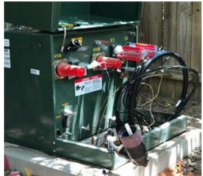
New cable in conduit with new transformer
