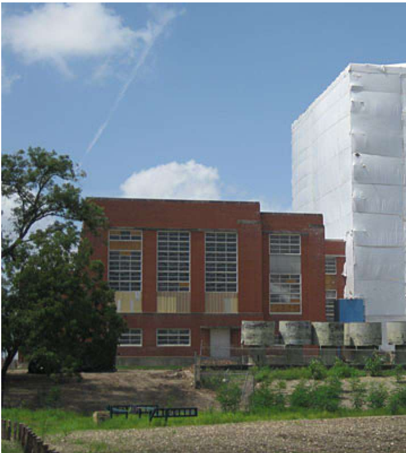
A giant white sheet hangs over part of Mission Road Power Plant.
