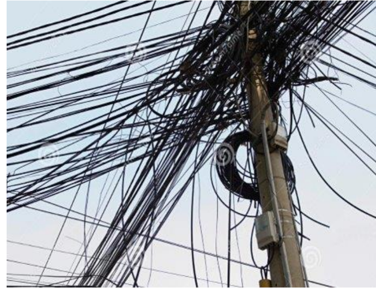
Pole with comms wires attached
