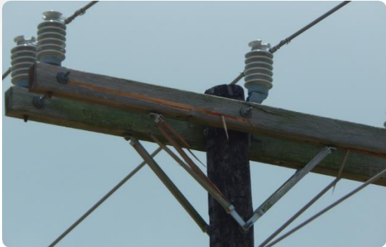
Lightning – damaged cross arm
